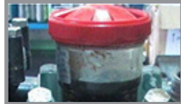
Oil in Functioning Pump
