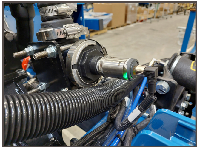
Sensor at the pump flow line
