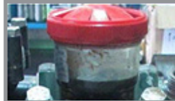
Oil in Functioning Pump
