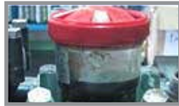
Oil in Functioning Pump
