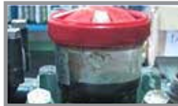
Oil in Functioning Pump
