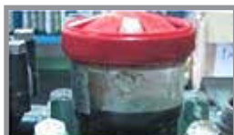
Oil in Functioning Pump
